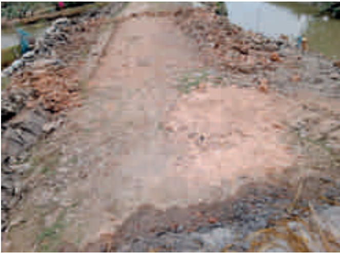
CC Road constructed at Boyermari Gram Panchayat in Sandeshkhali I Mandal, 24 Parganas through VCG efforts
